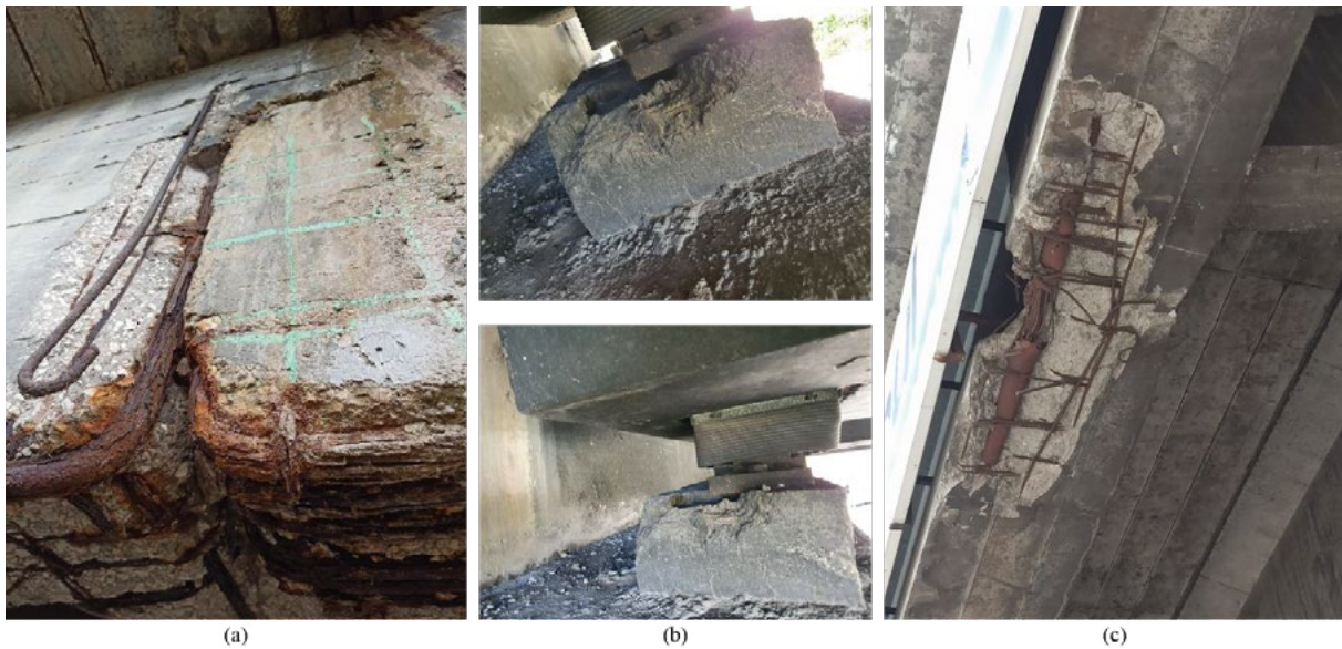
Fig 2. Example of significant defects: (a) deterioration of the Gerber support, (b) damage of supporting pad and (c) impact damage on prestressed reinforced concrete beam.
