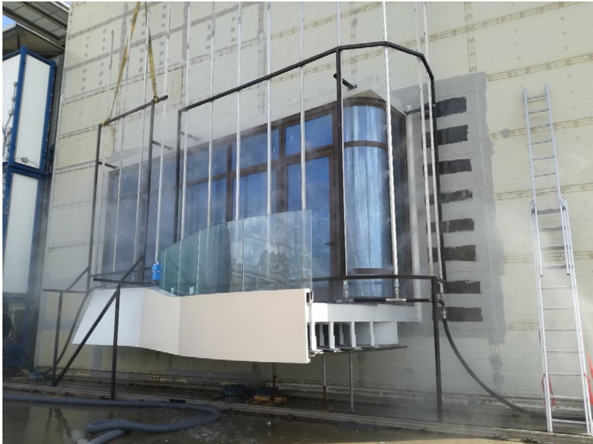
Fig 2. Water bomb test on curtain wall, according to ASTM E331-00 (2009). (Credit: Martino Milardi, 2020)
