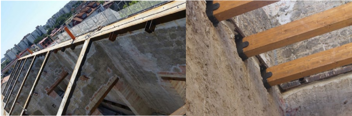
Fig 3. Casalnuovo (Na), Lancellotti Palace, structural intervention details a) The ribbing of the pitched roof; b) beams reinforced with special metal curb (which don't require breaking the wall).
