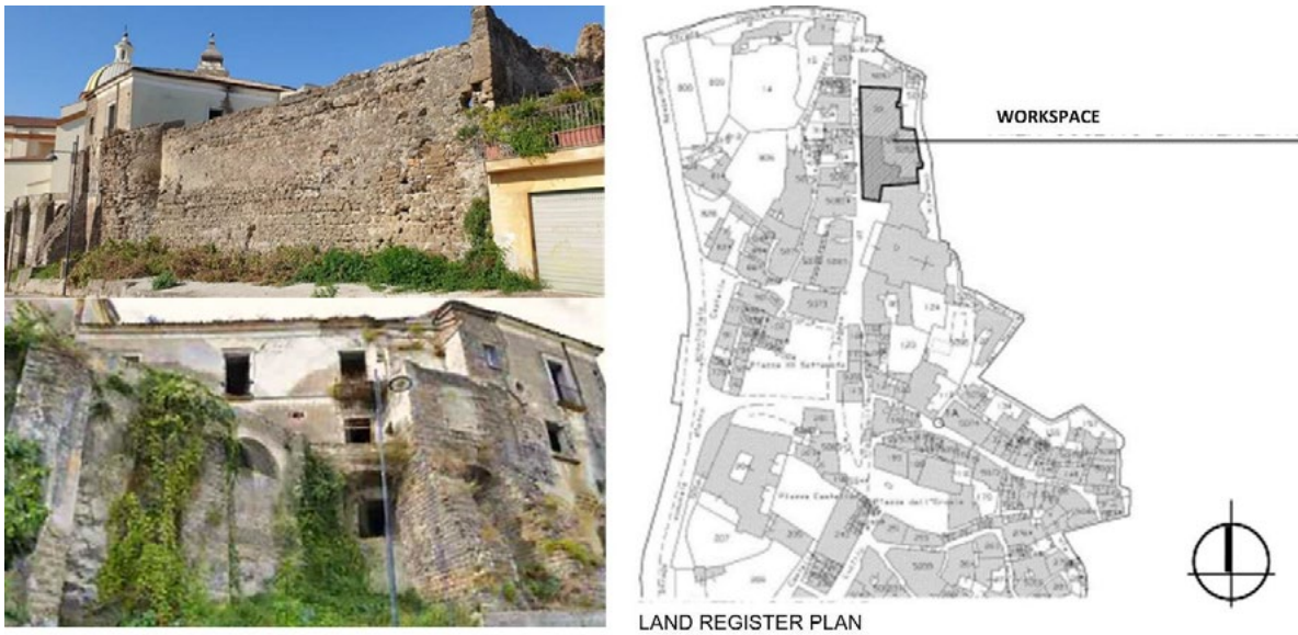
Fig 3. Back façade of the AGP structure attached to the church and the medieval boundary wall (credit: A. Maio)
